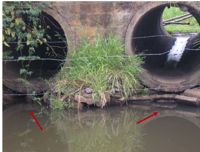
Arrows pointed erosion under gallery (Type 4)
