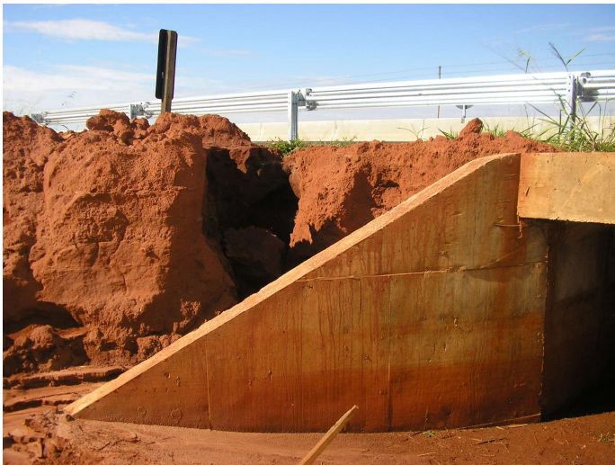
Area with severe erosion on slopes (Type 5)
