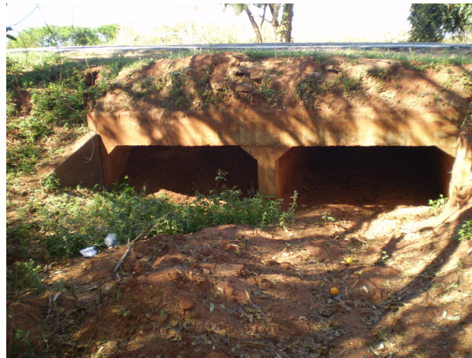
Rainwater gallery with two cells silted (Type 1)
